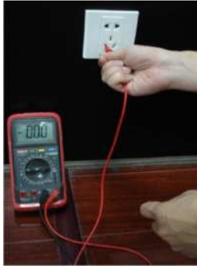
Appendix Figure 7-7 Check neutral cable connection
