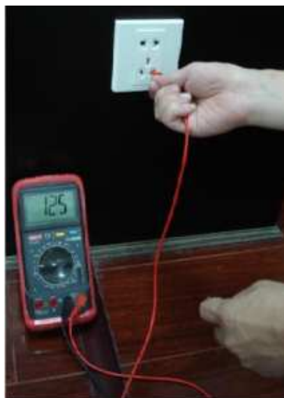
Appendix Figure 7-6 Check live cable connection
