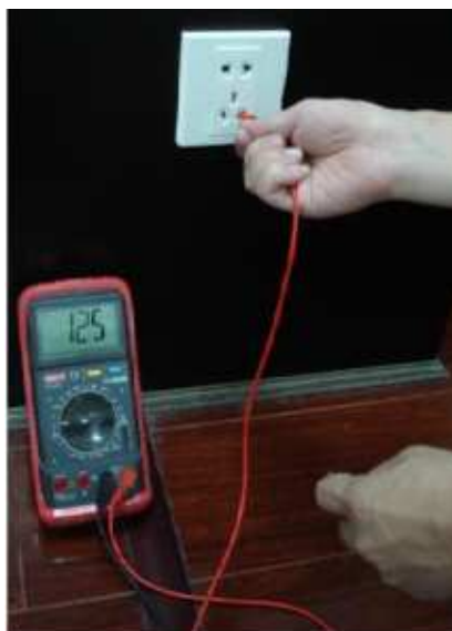
Appendix Figure 7-6 Check live cable connection
